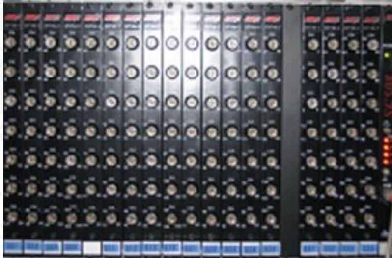
Figure 30. View of a full crate housing 420 HV channels.
